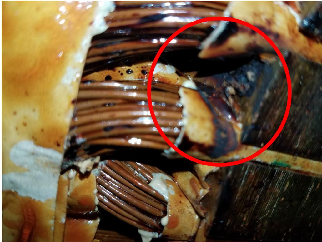
Coil that shorted to ground at edge of laminations
